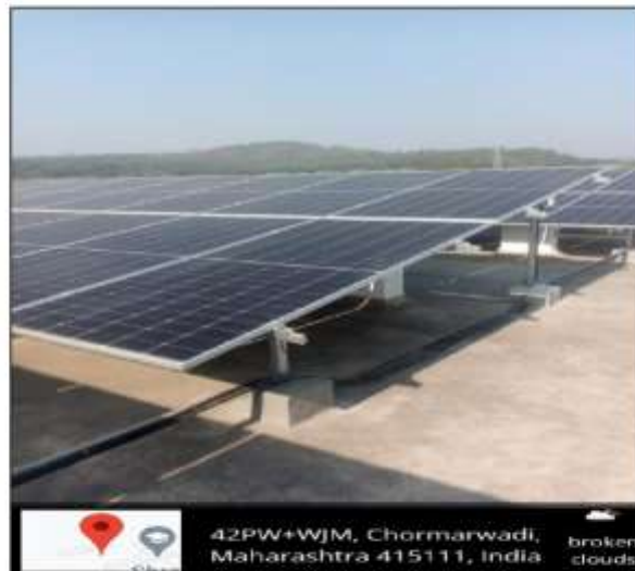
Photograph of Roof Top Solar PV Plant:
