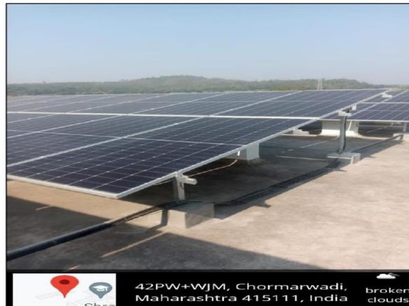
Photograph of Roof Top Solar PV Plant:
